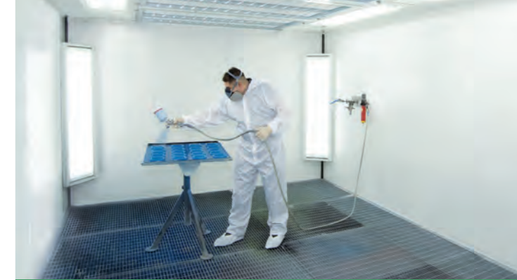
In-house lacquering facility
